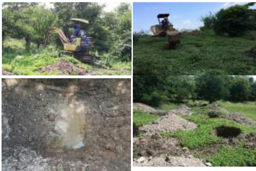
Figure 1 a, b) Preparing plot site with Caterpillar c, d) hole and hole line in the plot.
