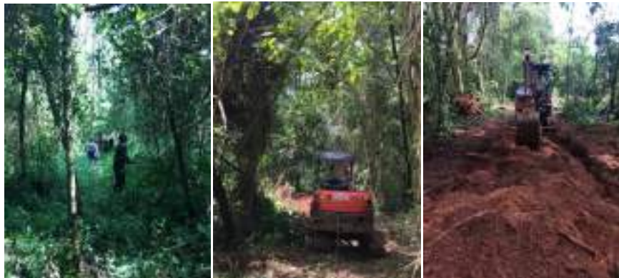
Figure 1 a) Man power line opening b) Clear area by Caterpillar, c) Soil loosening
