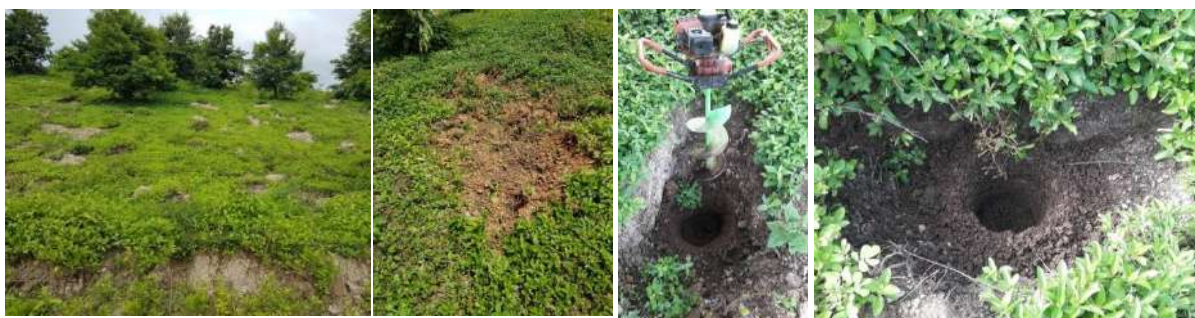
Figure 2. planting holes were dug by using backhoe and loosening lower soil using soil driller..
