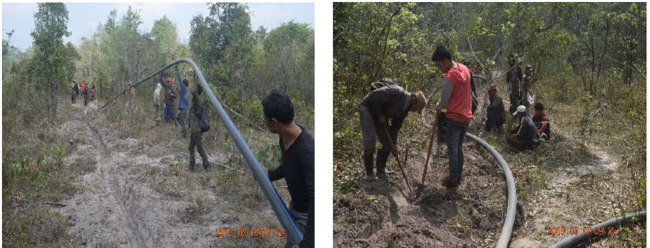
Figure 16. Running pipes from water tank in Kongtoun Mountain to water tank in Kongtoun village
