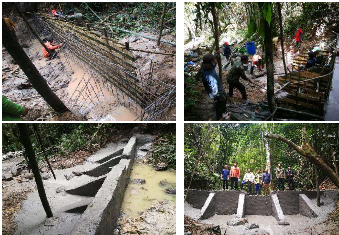
Figure 19. A small check dam in Phoukhaya mountain near the enrichment plantation site
