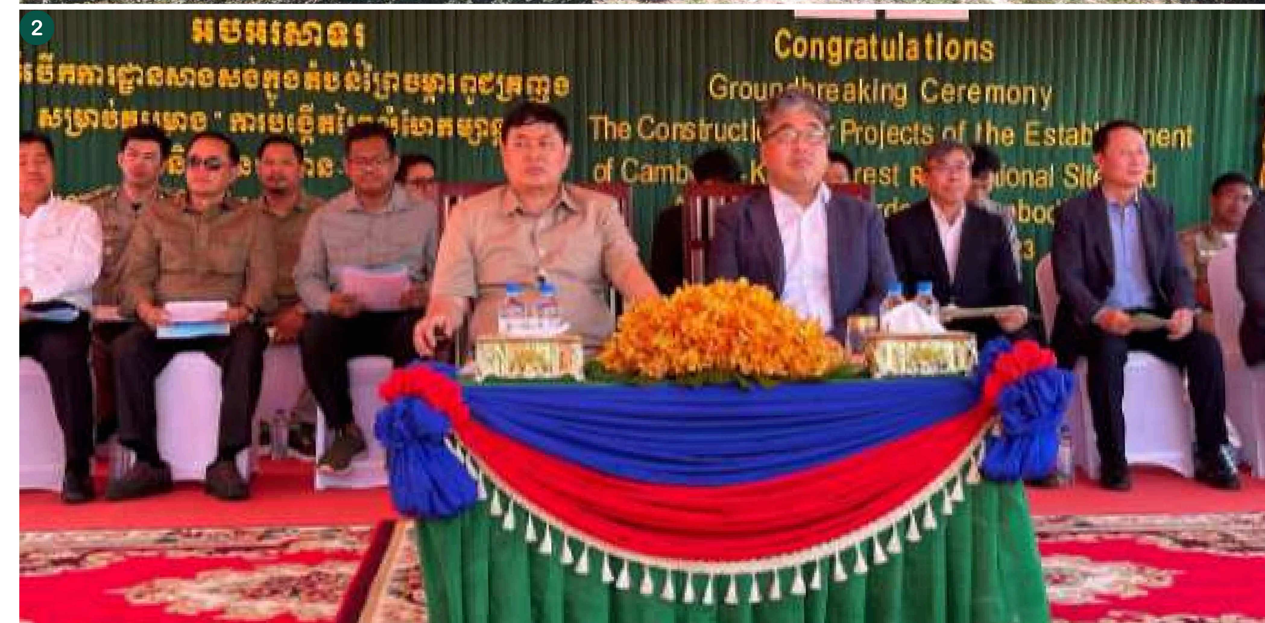
1. Site clearance for ASEAN-Korea Garden construction, in Khun Ream commune, Banteay Srei District, Siem Reap province 2. Groundbreaking Ceremony in Khun Ream commune, Banteay Srei District, Siem Reap province
